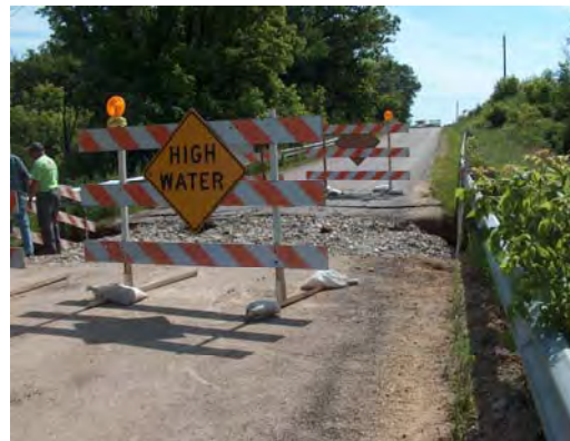
New Haven Flood Damage
