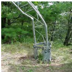
Wind Damage - Com. Tower
