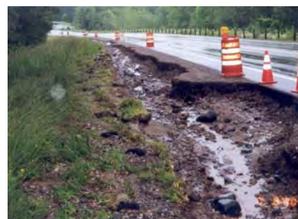
Flood Damage. US Hwy 8
