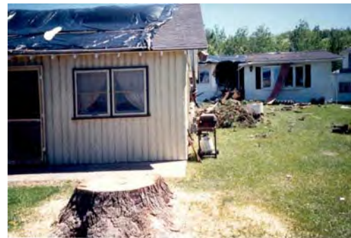
Tornado Damage, Forest County
