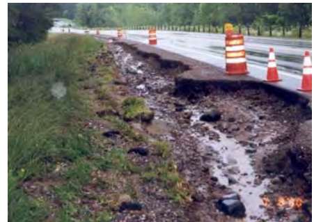
Flood Damage. US Hwy 8
