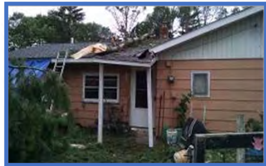
Straight-line Wind Damage, Armenia 2015
